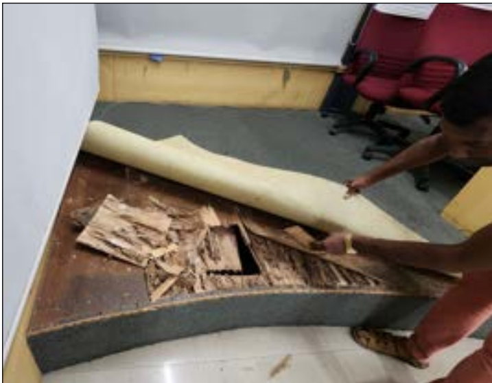
CEC HALL DIAZ PLATFORM COMPLETELY DAMAGED
